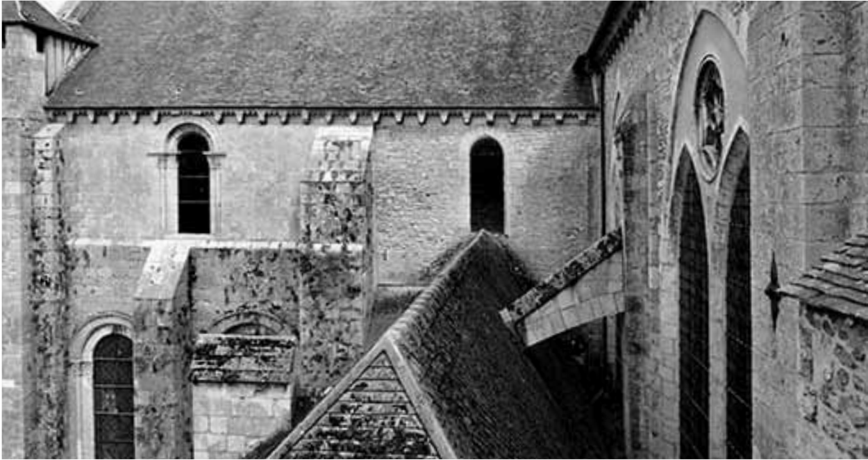
Rubble wall in first bay of north transept and the north wall of the nave
