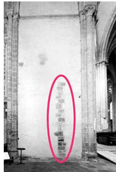
North side of north wall, east bay of choir, with the outline of an intended side chapel outlined.
