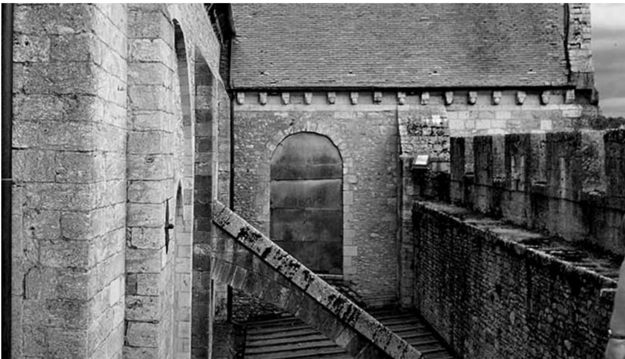
Rubble wall in first bay of south transept and south wall of the nave
