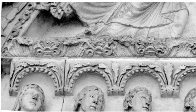
Upper south lintel, left canopies. The joint is clearly visible from this angle
