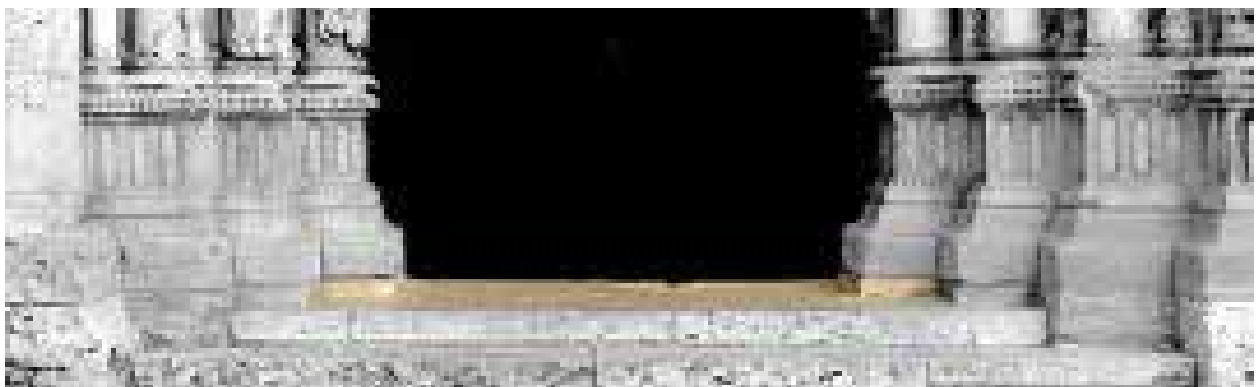
North door with upstands marked at each end of the threshold to locate the plinths.
